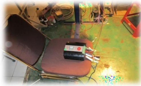
Figure 5: Shows the controller of wind turbine and PV.
